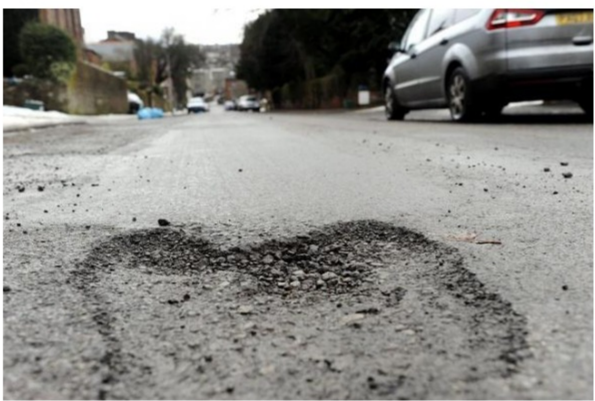
The UK has a pothole backlog that could take 11 years to repair
